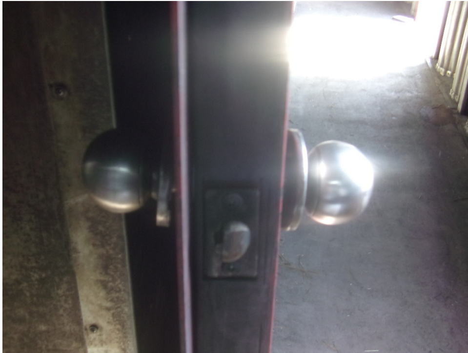
Damaged knob at hollow metal door between Hallway 202 and Room 204
