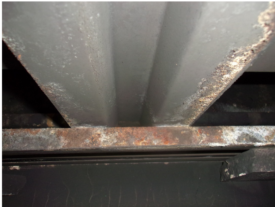
Minor corrosion on hat channel where Padgenite panel was removed for observation at ceiling in Burn Room #1
