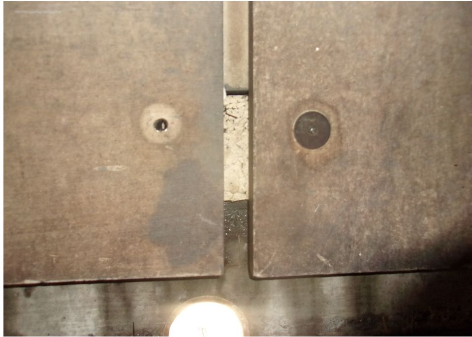
Typical missing screw and washer at Padgenite panels at burn room ceilings and walls
