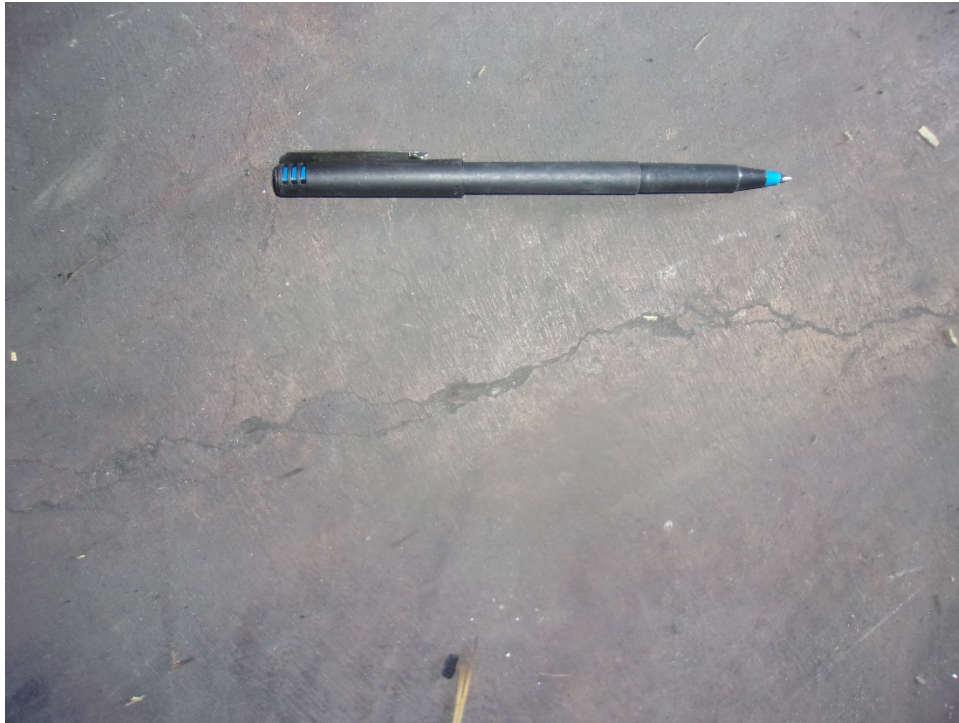
Typical minor cracks in concrete topping at elevated floors
