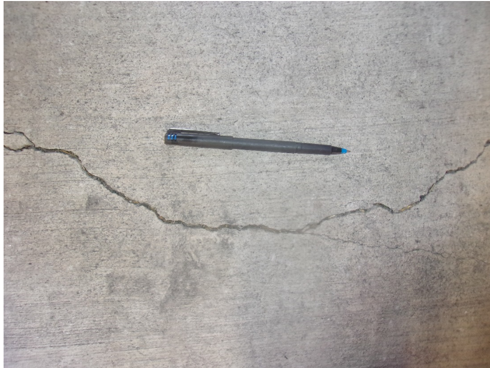
Typical minor crack in concrete slab-on-grade
