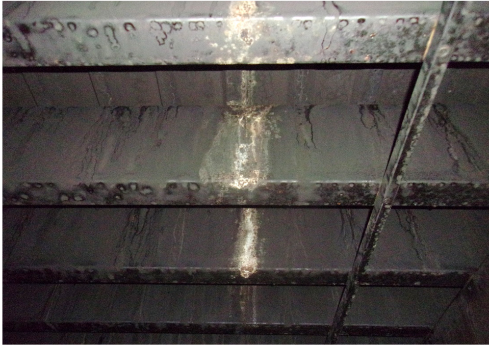
Minor staining on steel framing at ceiling in Room 101
