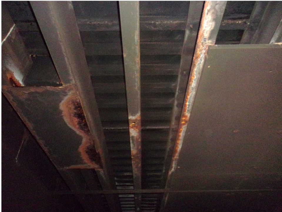
Corrosion on steel framing at ceiling of Room 204 beyond rollover lining outside door opening into Burn Room #2
