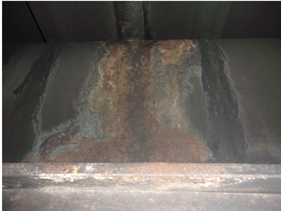
Minor corrosion on steel framing where Padgenite panel was removed for observation at ceiling in Burn Room #1
