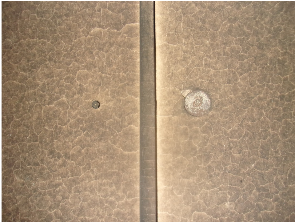
Missing washer at screw (at left in photo) at Padgenite panel at east wall in Burn Room #1
