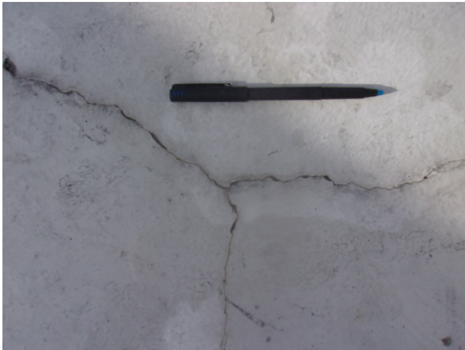
Typical minor cracks in painted concrete topping at flat roofs
