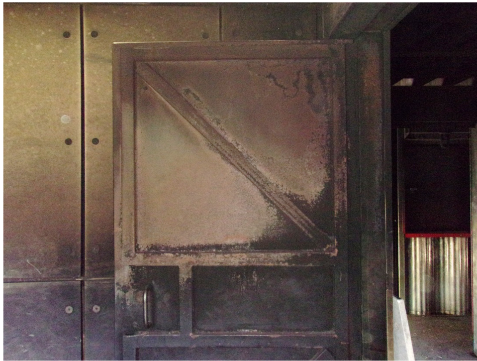
Corrosion on steel plate door at west side of Burn Room #2
