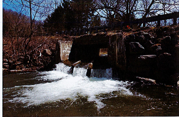
Before 2 Plunge pool and fish passage barrier
