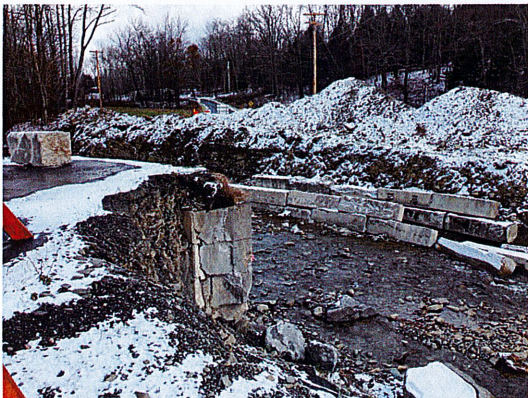
Before 2 Bridge out! Town purchase double box to replace it, but unable to get NYSDEC permit.
